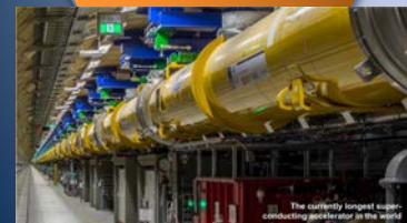
The currently longest superconducting accelerator in the world
