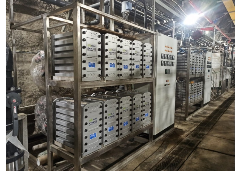
Water system is almost ready for commissioning
