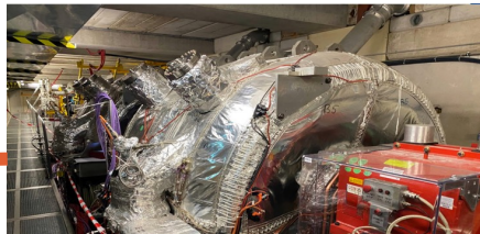
Outdated LLRF and HLRF for C10 cavities
