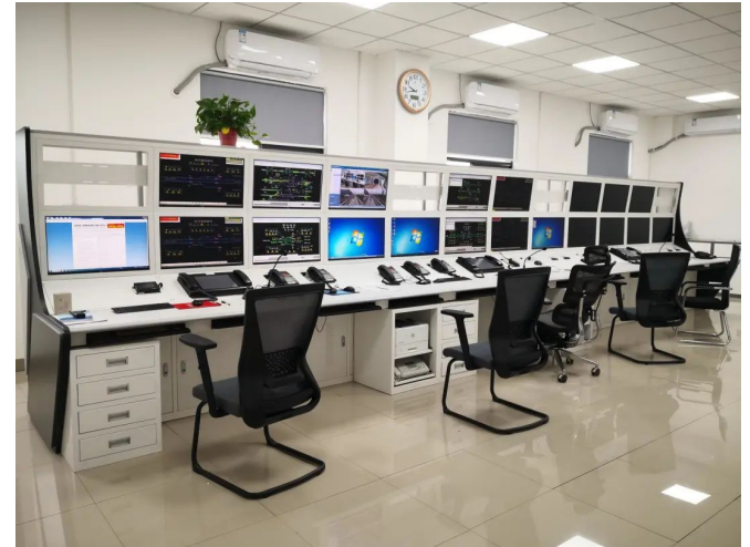
Train Operation Command Room of Deqing Hefei-Hangzhou Railway Depot
