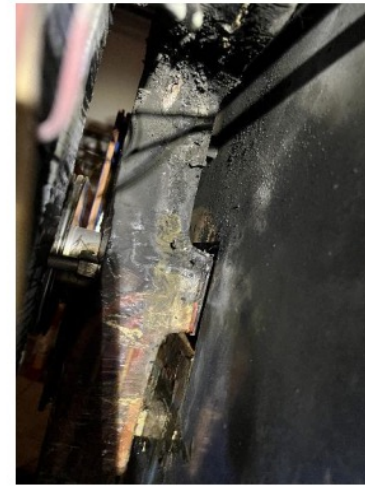
Connection side coil
