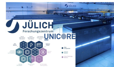
The Jülich Supercomputing Centre operates one of the most powerful supercomputers in Europe, JUWELS, and JUNIQ the first European infrastructure for quantum computing. UNICORE offers seamless access to the Supercomputers.
