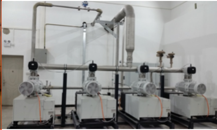
2K pumping system
