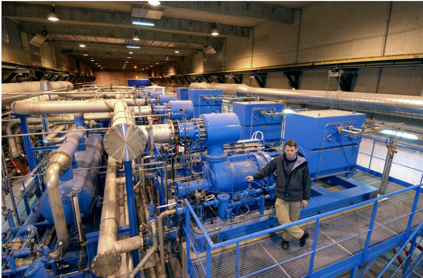
LHC 1.9 K cryo plant
