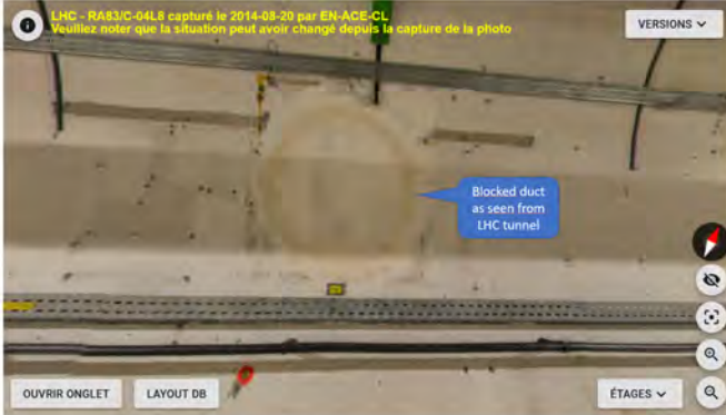
Figure 4 — Duct for MAPP Outrigger location, seen from LHC tunnel
