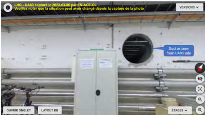
Figure 5 — Duct for MAPP Outrigger location, seen from UA83
