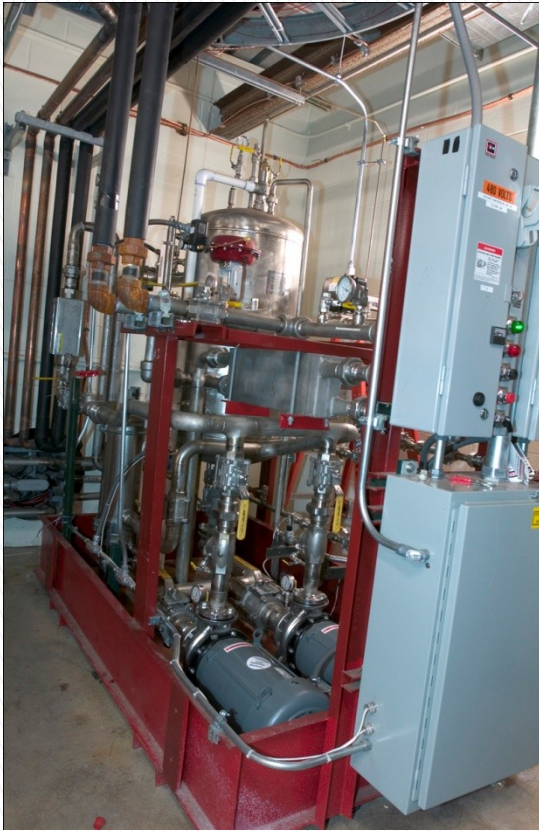
Radioactive Cooling Water Systems
