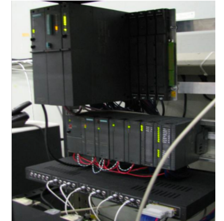
ECAL Safety System (Run 1 & Run 2)
