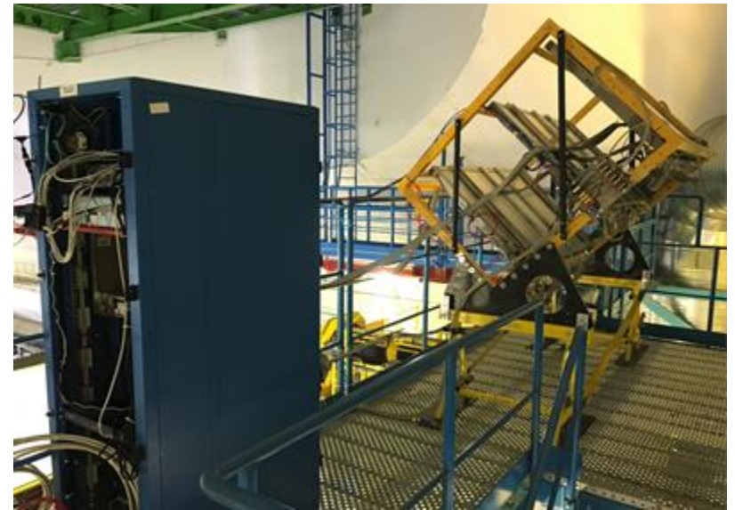
proANUBIS + DAQ rack installed in their positions within the ATLAS experimental Cavern ( ATLAS Side A Level-12 of UX15 )
