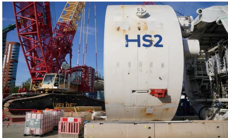
A tunnel boring machine at the HS2 site near Old Oak Common in west London. Photograph: Jonathan Brady/PA
