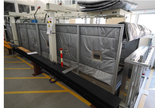
Existing Diamond oven
