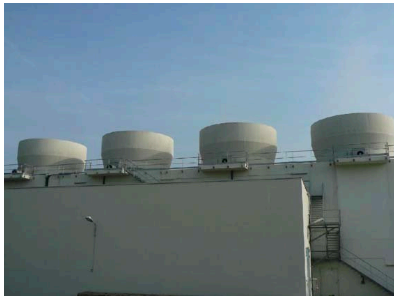
Cooling towers at CERN
