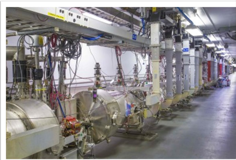
Superconducting RF Linac (1.09 GeV per straight-away)
