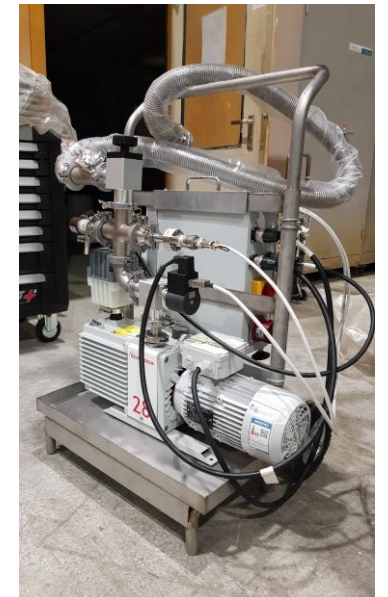
M2 New Pumping Group
