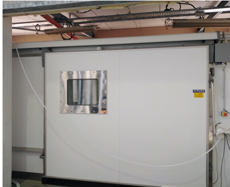
Climate Chamber functional To do: Need feedthrough for cables and CO 2 lines
