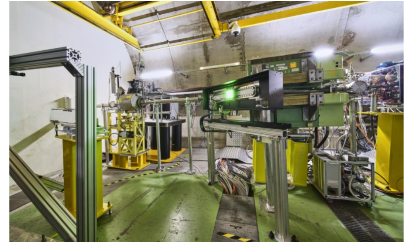
AWAKE facility, with separation wall to CNGS target area on the left
