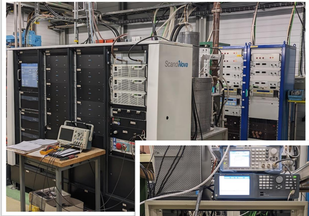
Modulator and S-band 40MW klystron (above)
