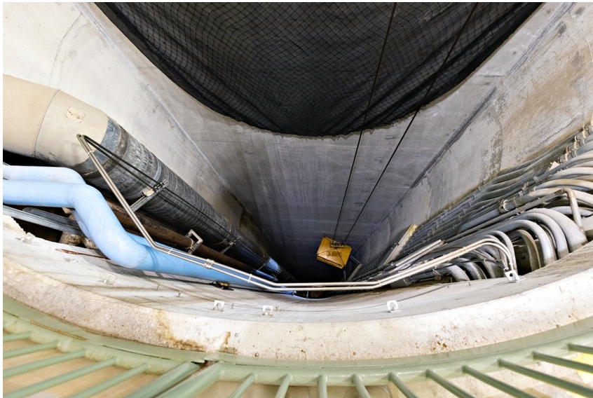
Existing personnel basket in use.
