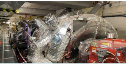
Outdated LLRF and HLRF for C10 cavities
