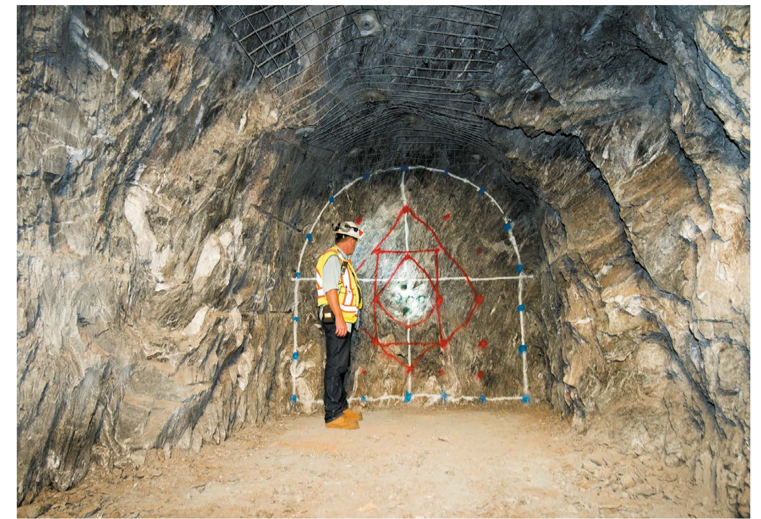
An underground test blast area for the DUNE neutrino experiment in Lead, South Dakota.
