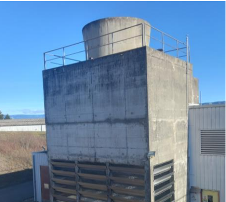
Outdated (and not very "green") cooling and ventilation systems
