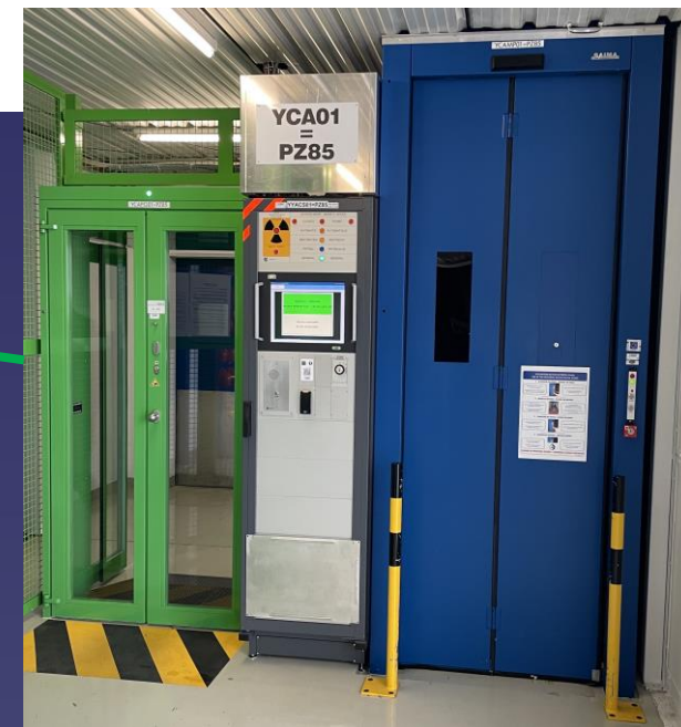
Standard LHC Access Control System (LACS) door. Probably a lightweight solution could be installed at the top platform of PX46, since access to the AI will NOT be an access to the LHC . Availability and use of oxygen-generating self-rescue masks to be assessed
