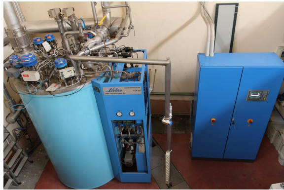
LINDE He refrigerator/liquefier
