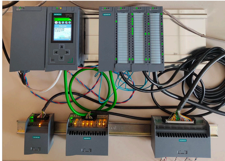
Figure 3. Siemens programmable logic controller setup used for the Environmental stress screening system, in order to independently monitor temperatures inside all 12 boxes using PT1000 sensors and to provide safety interlocks to power supplies in case of over-temperature, enabling safe unattended operation of the system. The system is based on the design of the safety system that will be installed at the upgraded CMS experiment and provide safe operation of the EB detector during the operation of the HL-LHC.
