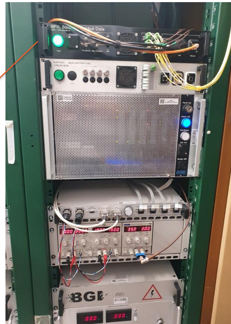
Back-end, PLC and power supplies
