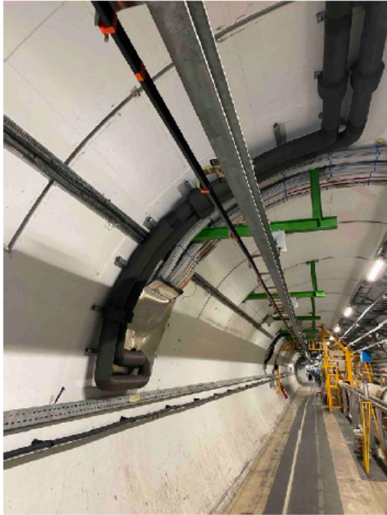
Cables are available, as well as the rail for transporting the apparatus
