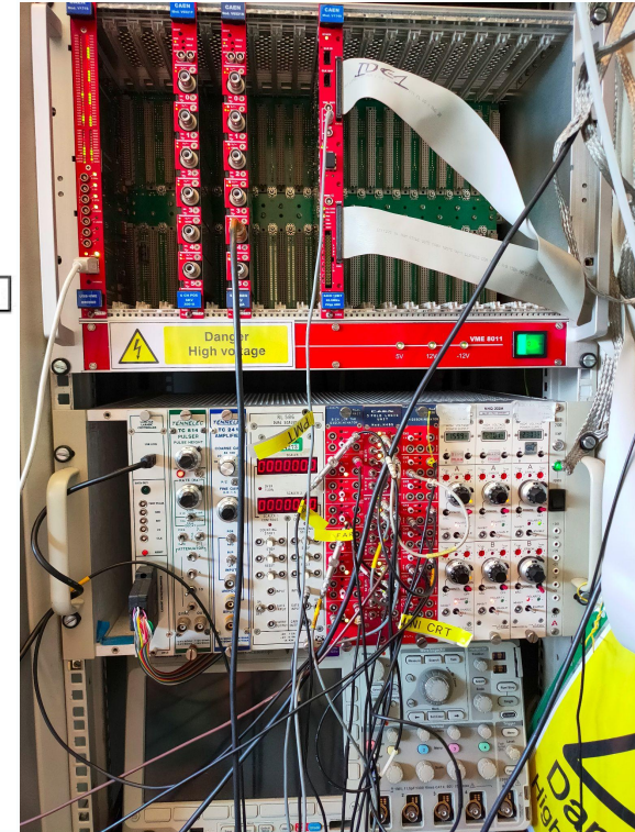
STEEL rack: CAEN-V6521 voltage supply (top), logic trigger system (middle), oscilloscope (bottom).
