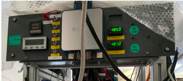
Live LAr pressure and LAr/LN temperature monitors above STEEL. LAr pressure is calculated using a partial differential pressure monitor.
