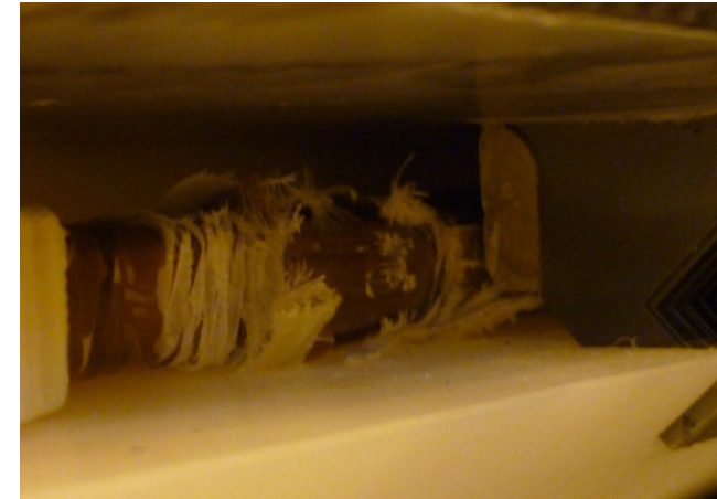
Dipole line MQ double lyra Kapton damaged
