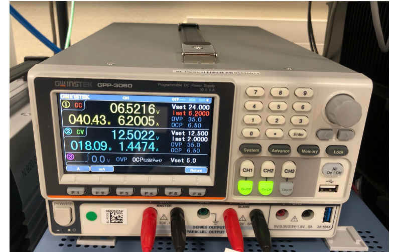
Cooling water tank PSU for the fan and the water pump
