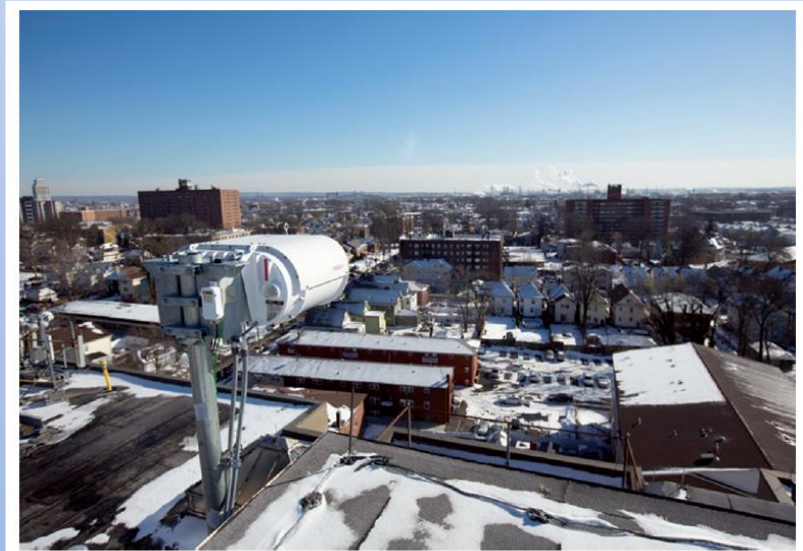
Laser units on rooftops connect New Jersey's Nasdaq data centre with the New York Stock Exchange.
