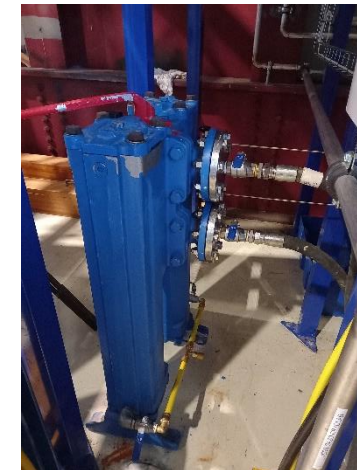
2. Cold box water inlet filter
