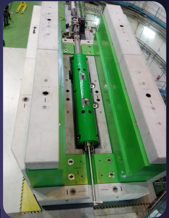
SPS Internal Beam Dump (shielding open)
