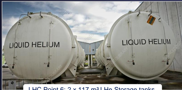
LHC Point 6: 2 x 117 m 3 LHe Storage tanks
