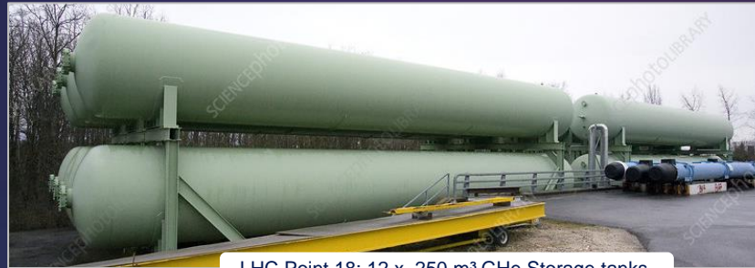
LHC Point 18: 12 x 250 m 3 GHe Storage tanks
