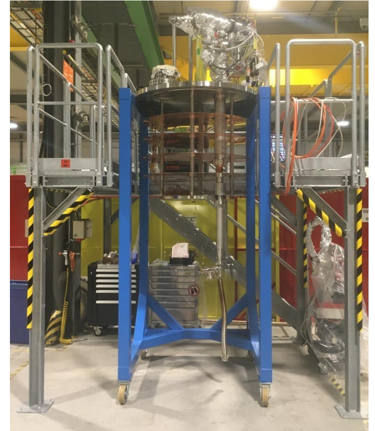
New V4bis insert and preparation area
