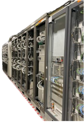
HL-LHC 18kA PC with Energy Storage (Battery) Systems - Proto
