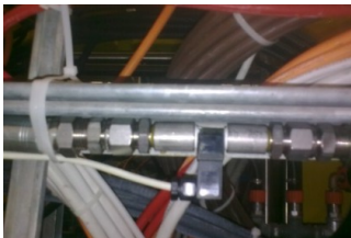
Turbine flow meter
