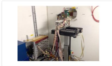
Control room patch panel view
