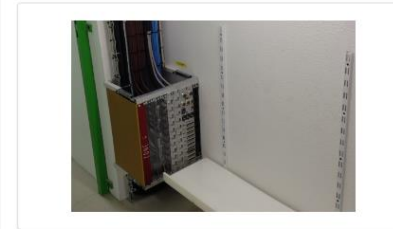
Control room patch panel view
