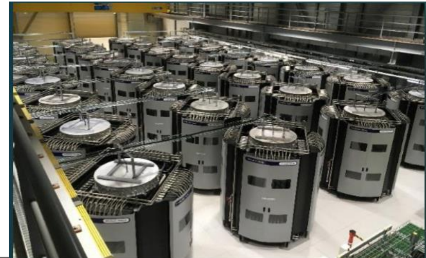
Solid State Power Amplifiers at the CERN PS
