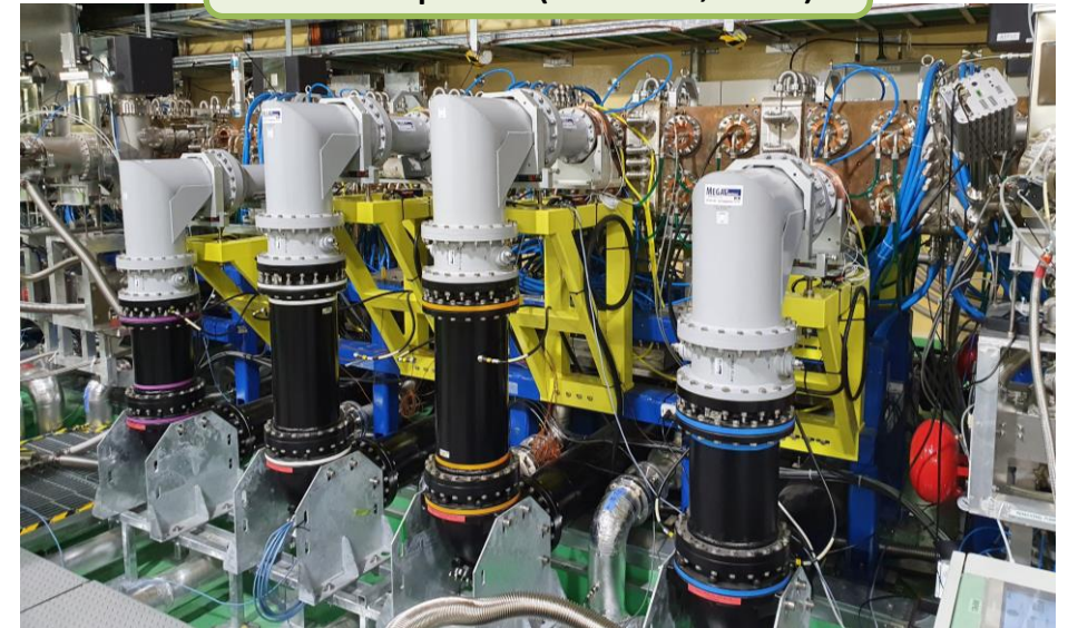
4 of the 8 coaxial lines supplying RF to RFQ
