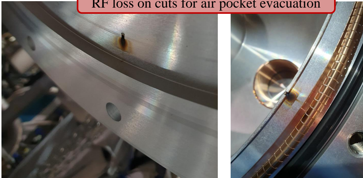
RF loss induced heat in the cuts used for evacuation of air pocket near O-ring.
