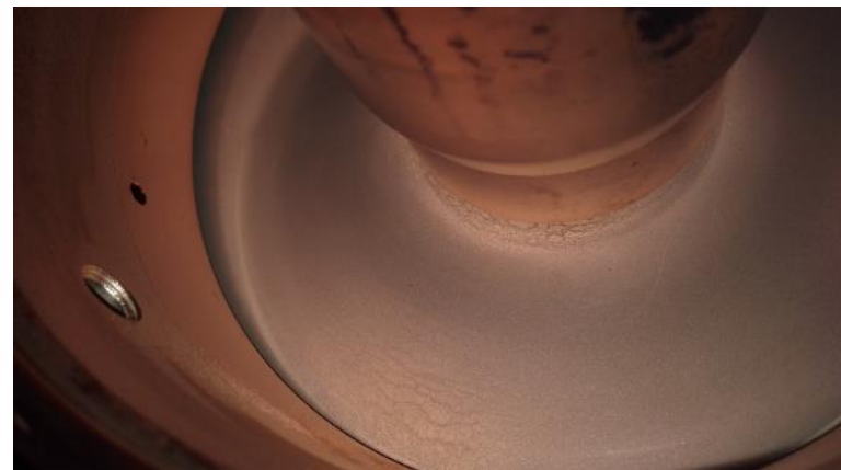
2#: Window cracked due to disabled ARC interlock (BEPCII 500MHz SCC)
