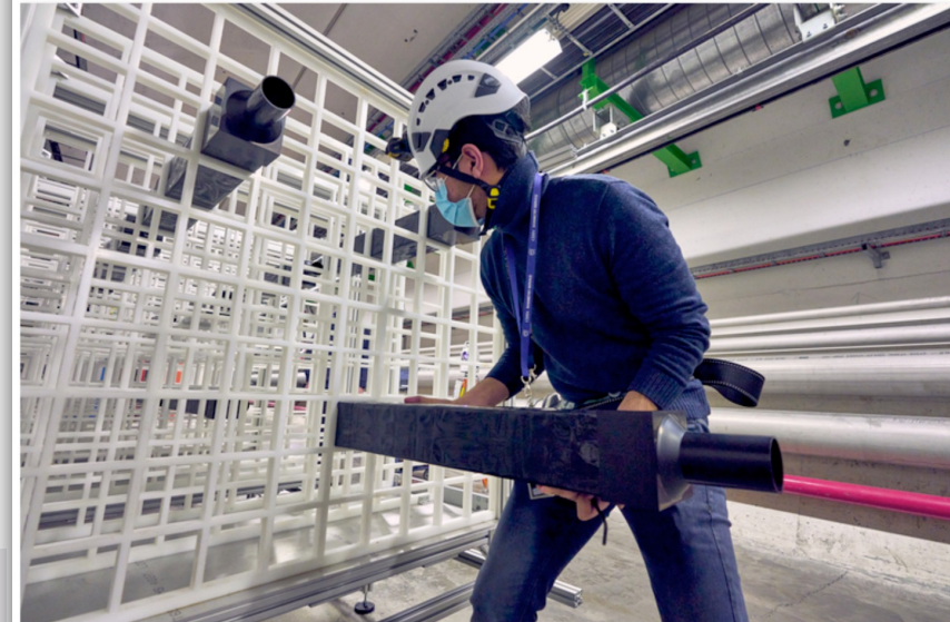
Installation of the support structure for the MAPP detector components. (Image: CERN)
