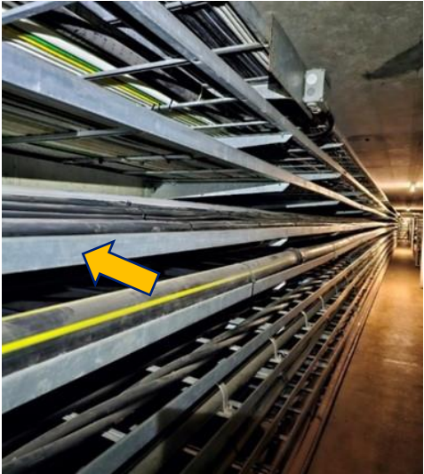
Overloaded cable tray, EDMS: 2900780
