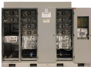
Power converter (photo HL-LHC)
