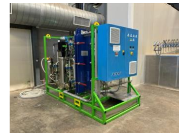
L3 Power Converter Cooling Plant
