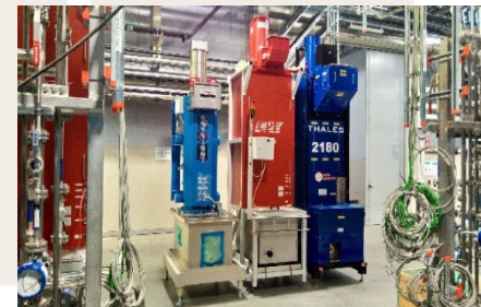
Klystrons used at ESS
