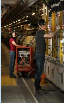
Quality Control of superconducting electrical circuits ELQA TEAM
