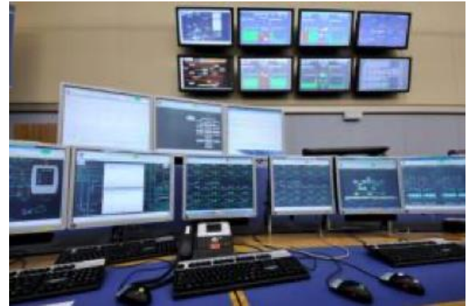
CERN CRYO Central Control Room
