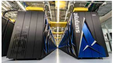
IBM Summit 2018 200 PFLOPS 873 m 2 , 13 MW 219 kms of cabling
